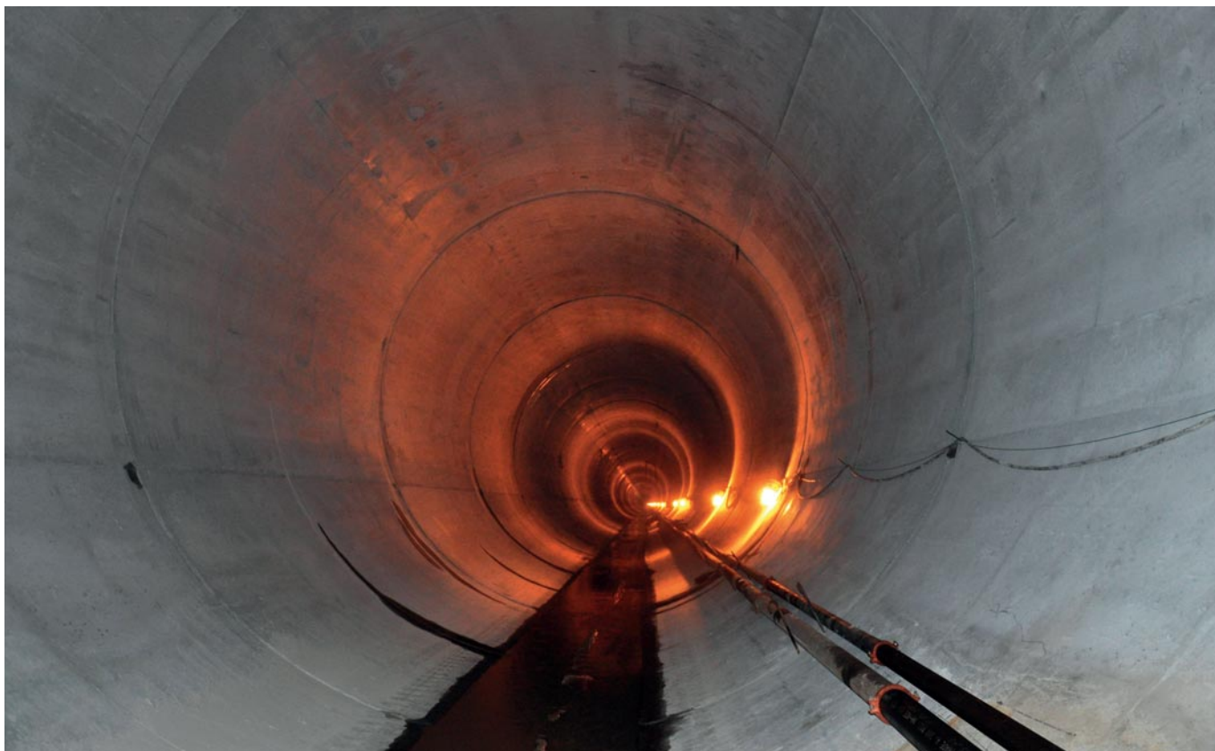
A defect free concrete surface improves the longevity of the sewer system
