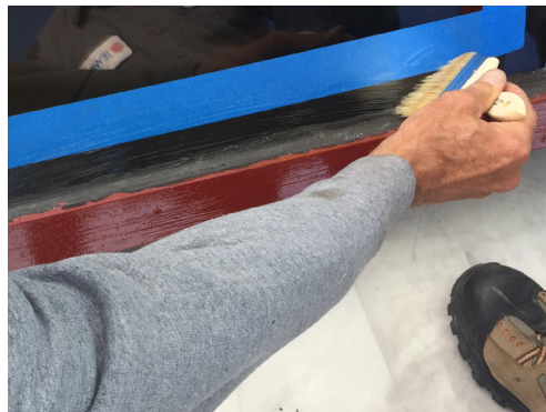
Prime frame and mullion with Sikalastic® EP Primer/Sealer. Mask off skylight 2 inches from the mullion and prime glass with Sikalastic® Clearglaze.
