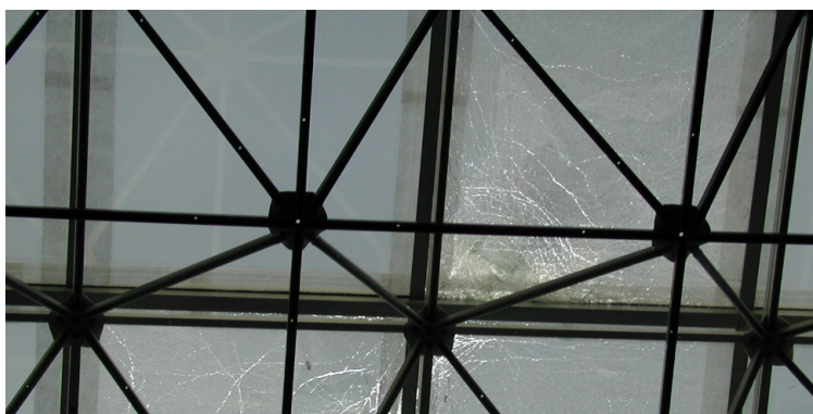
Skylight was protected with Sikalastic® Clearglaze. After a hurricane event, the skylights shattered but remained in place
