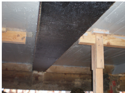
Girder after application of CFRP. Slab after application of epoxy coating. Note areas of shoring required comeback and touchup.
