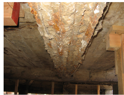
Extensive spalling of the beams, girders and slabs caused by severe corrosion of the reinforcing steel.
