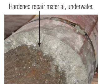
Hardened repair material, underwater. Cross Section of Repaired Pile. Repair Material Thickness = 1.5" - 2"
