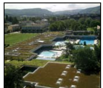
The first Sarnafil green roof was installed in 1969 and is still in place.
