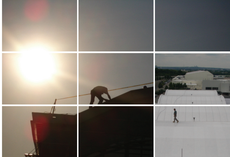
The Sarnafil Décor Roofing System being installed by Pioneer Roofing Systems on the Ronald Regan Washington National Airport Terminals B and C.
