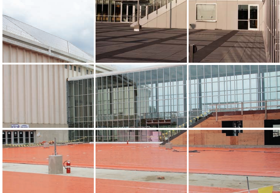
Sika Sarnafil's waterproofing membrane installed on the University of Northern Iowa's McLeod Center Plaza.
