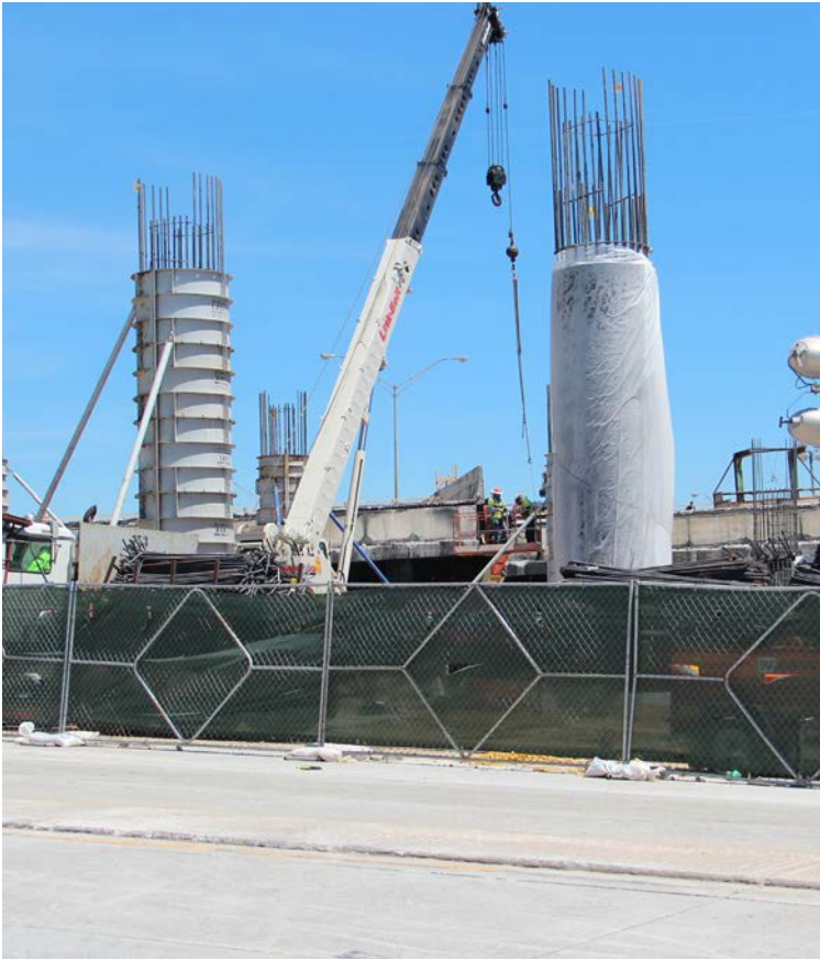
C.W. Matthews Contracting Company was chosen as the contractor for the repair
