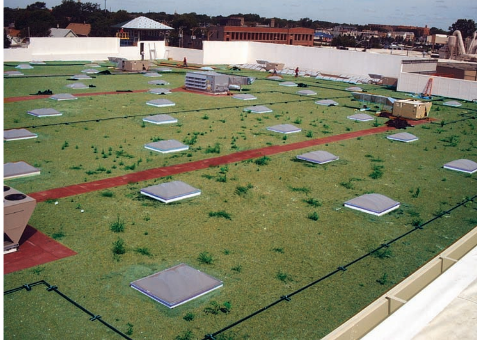
The vegetated roof atop the Wal-Mart in Chicago earned the company First Place in Sika Sarnafil's 2006 Waterproofing Project of the Year competition.
