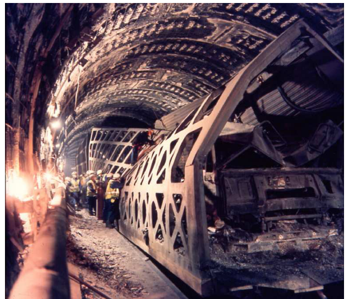
Figure 1. Channel Tunnel fire damage
