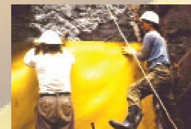
Ignoring substrate requirements and omitting protective backing materials
