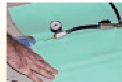
Physical testing of double welded seams and central void with compressed air
