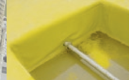
Garage roof deck with integrated tree planting box-outs; watertightness testing by flooding the plant boxes
