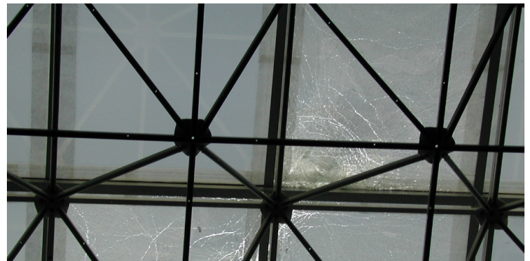
Skylight was protected with Sikalastic® Clearglaze. After a hurricane event, the skylights shattered but remained in place
