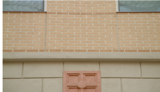
The block, accent medallion and running bond appearance (with darker stretcher bond accent rows), are all done in EIFS.
