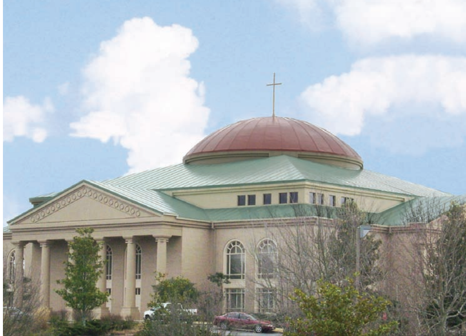
The Mount Carmel Christian School is finally watertight, thanks to the Décor Roof System. In addition to performance, the Décor system delivered style, with the roof having the appearance of a metal roof with standing-seam profiles.
