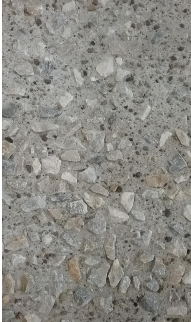
Figure 1: Concrete surface after MasterFinish EA 48 was rinsed and the surface was allowed to dry.
