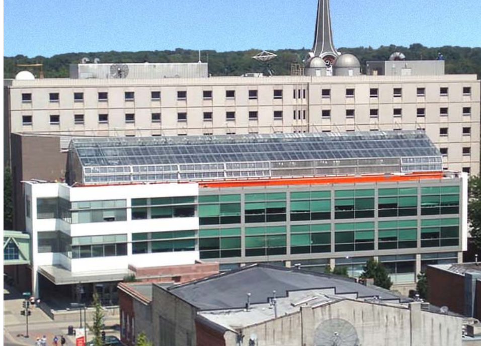
The 'Greenhouse Classroom' at the University of Iowa is located four stories up from street level in a highly congested area. Dryspace was able to lift the Greenhouse, install a new waterproofing system beneath it, and return it to its original location.
