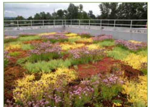
Tri-City Wastewater - Oregon City, OR
