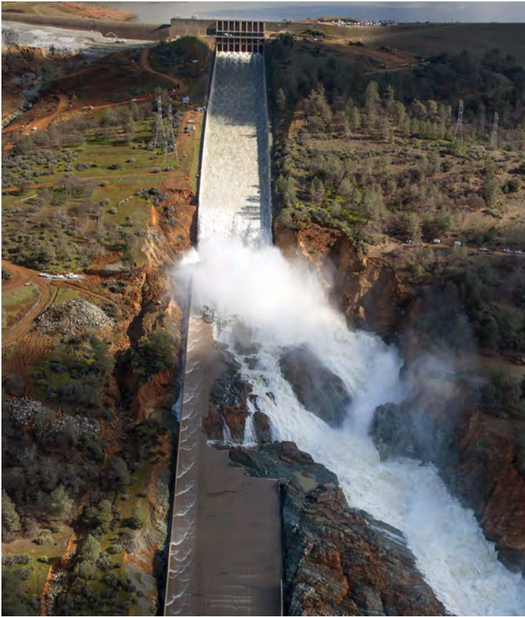
Oroville Dam spillway damage during failure
