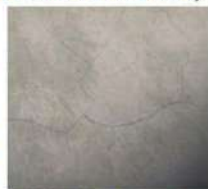
Fig. 3. Typical cracks in concrete
