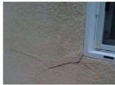
Fig. 1. Crack in exterior stucco
