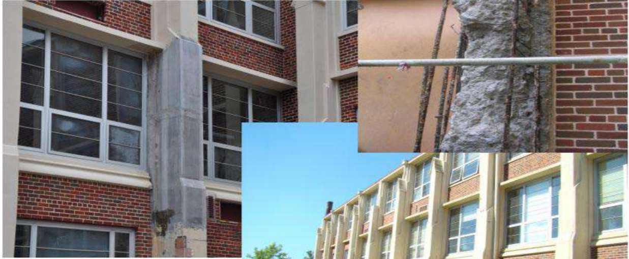
The figure and photos above show a typical repair detail and different phases of the repair process.
