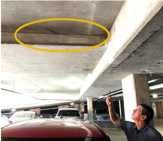
PT Slab Cracking
