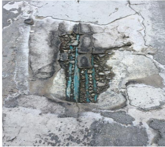
Low Concrete Cover
