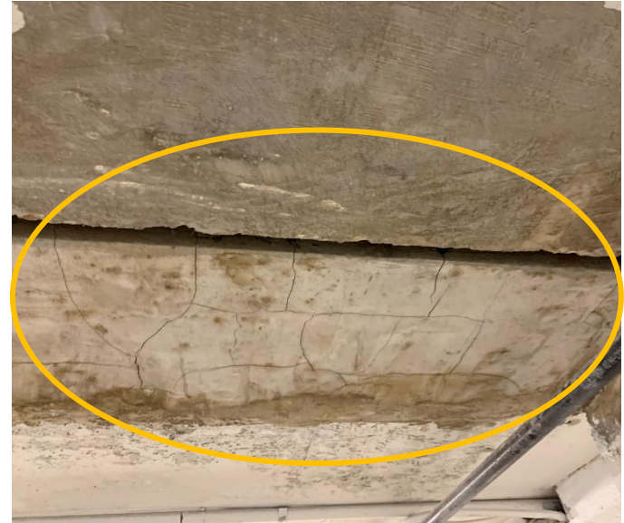
Garage Soffit Damage Under Expansion Joint
