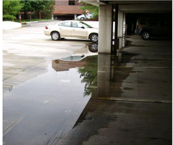
Poor Drainage/Clogged Drains
