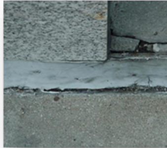
Concrete Joint Issues
