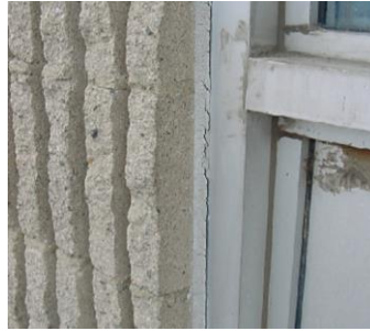
Concrete Joint Issues
