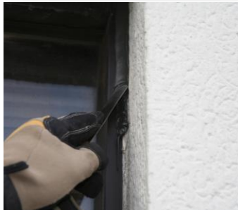
Improper Material Selection
