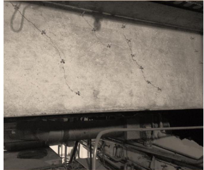
Beam shear Cracks
