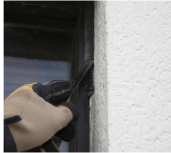
Improper Material Selection
