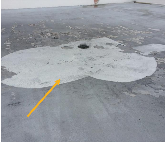
Failed Deck Coating
