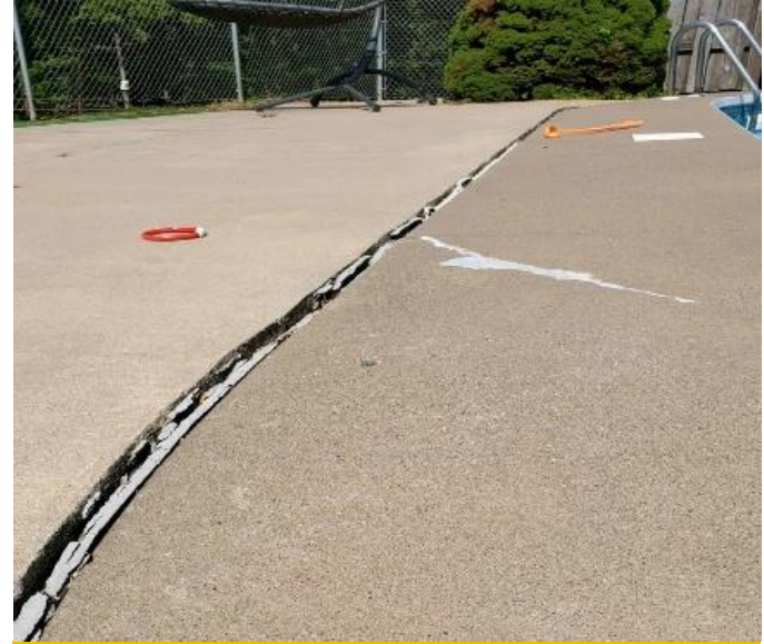
Joint Material Deterioration
