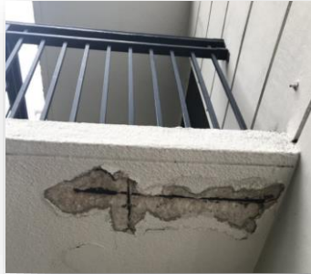
Low Concrete Cover
