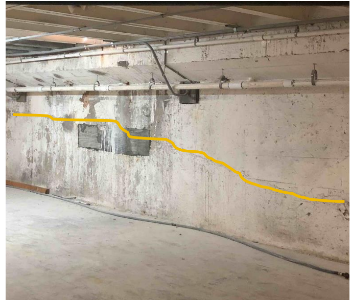
Pool vault wall cracking
