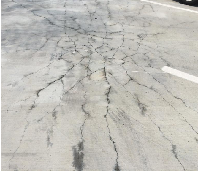
Punching Shear Cracks
