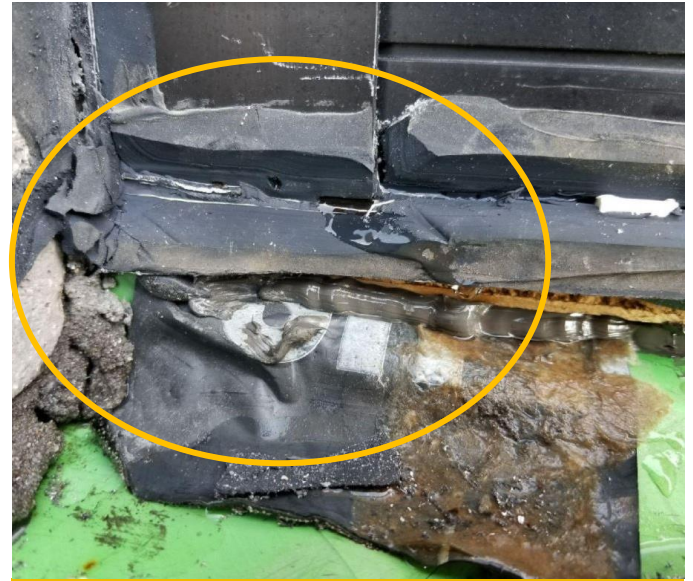
Window Flashing Failure
