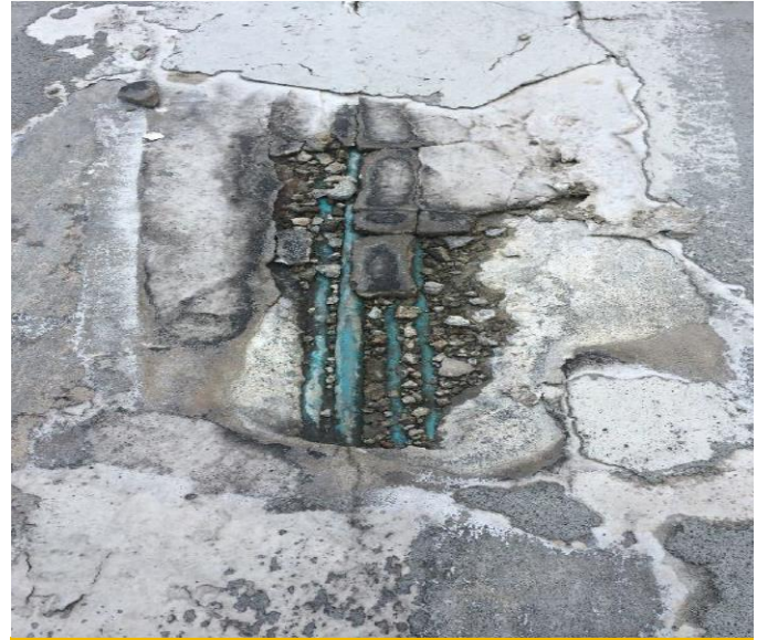
PT Exposure Due to Low Cover
