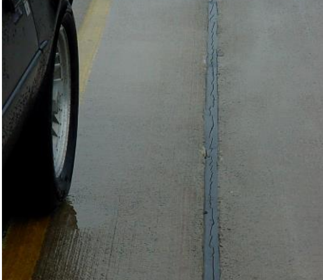
Failing Joint Sealant
