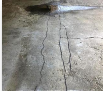
Concrete Joint Issues
