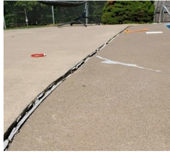
Concrete Joint Issues
