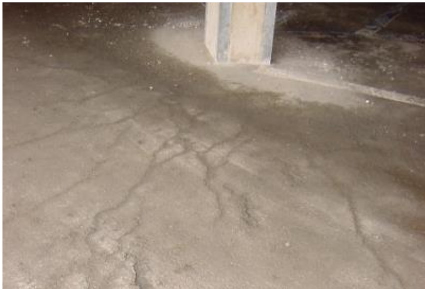
Punching Shear Cracks
