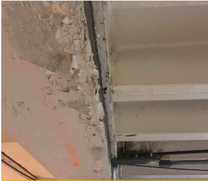
Water intrusion below pool deck
