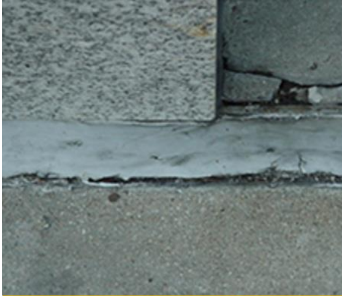
Joint Sealant Failure
