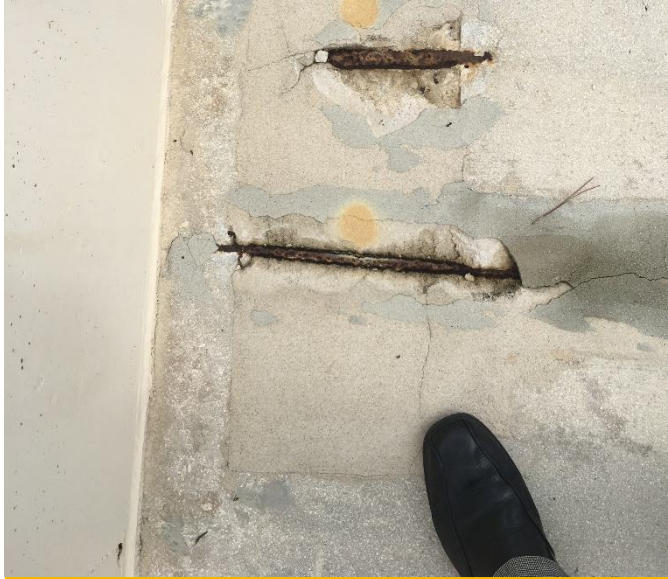
Parking Deck Spalling
