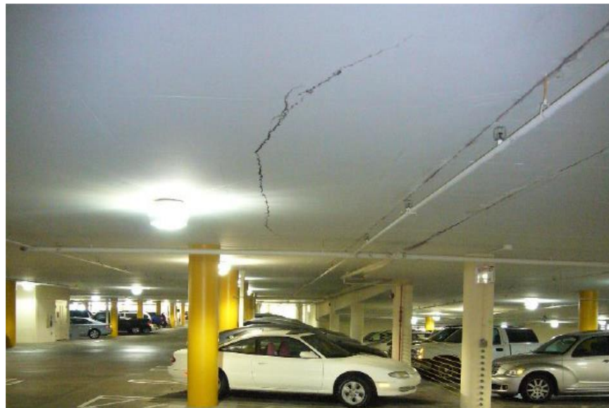
PT Slab Cracking
