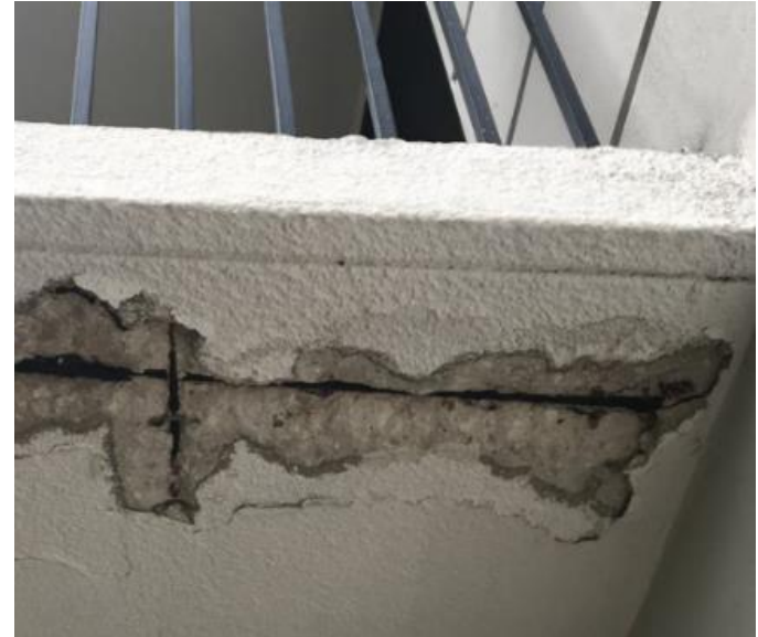
Concrete Spalling on Balcony
