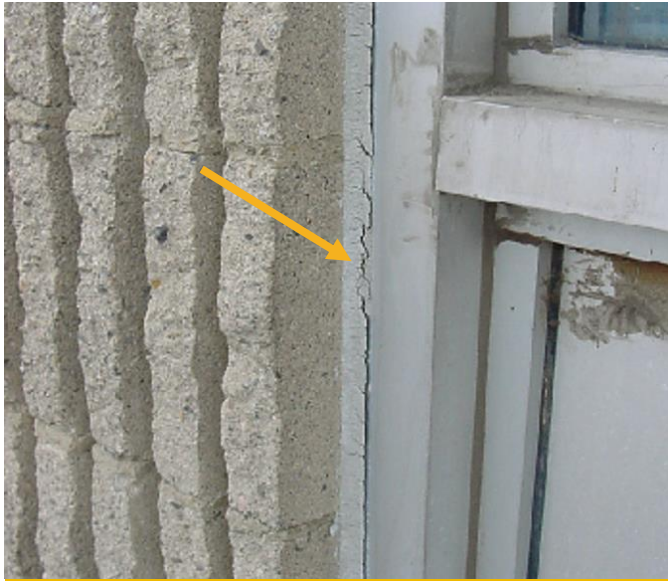
Adhesive Failure in Window Joint
