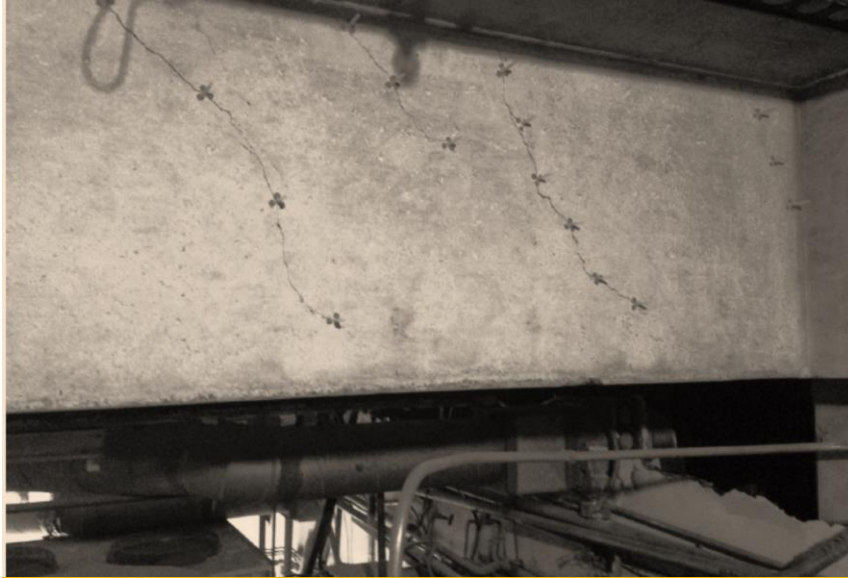
Shear Cracks on Beams
