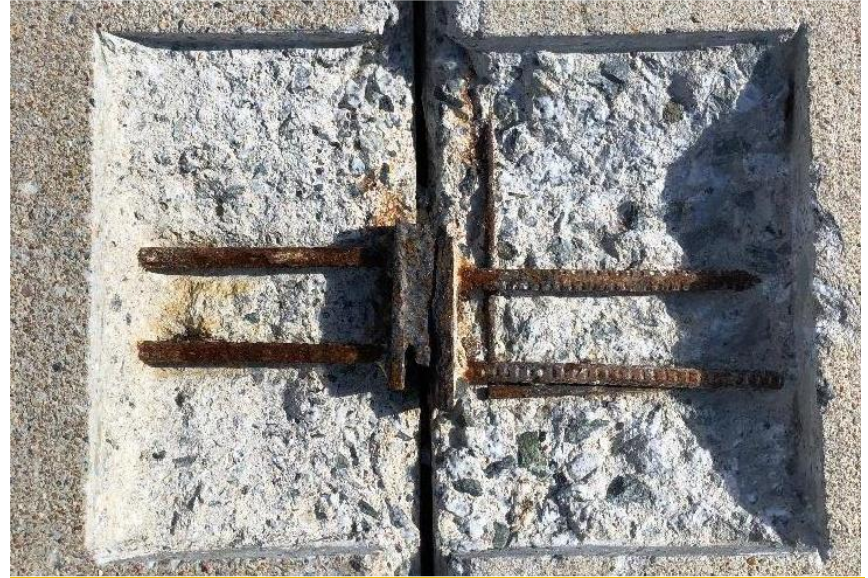
Double Tee Welded Connection Issue
