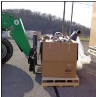
A gaylord filled with old vinyl membrane from the SuperTarget in Olathe is readied for shipment to Sika Sarnafil for recycling.
