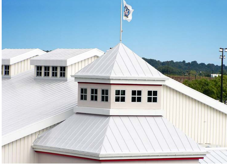
Pfister Roofing installed a Décor Roof System atop the Grandstand Paddock at the Meadowlands Racetrack in East Rutherford, New Jersey. The job won the roofing contractor third place in the Sika Sarnafil 2007 Project of the Year competition.
