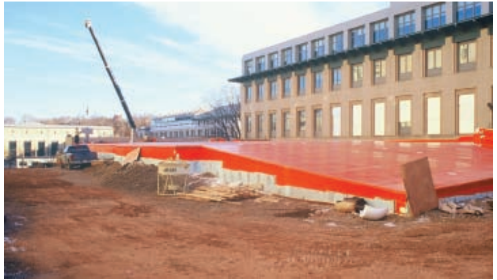
Sarnafil's G476 being installed on top of the building's concrete roof deck
