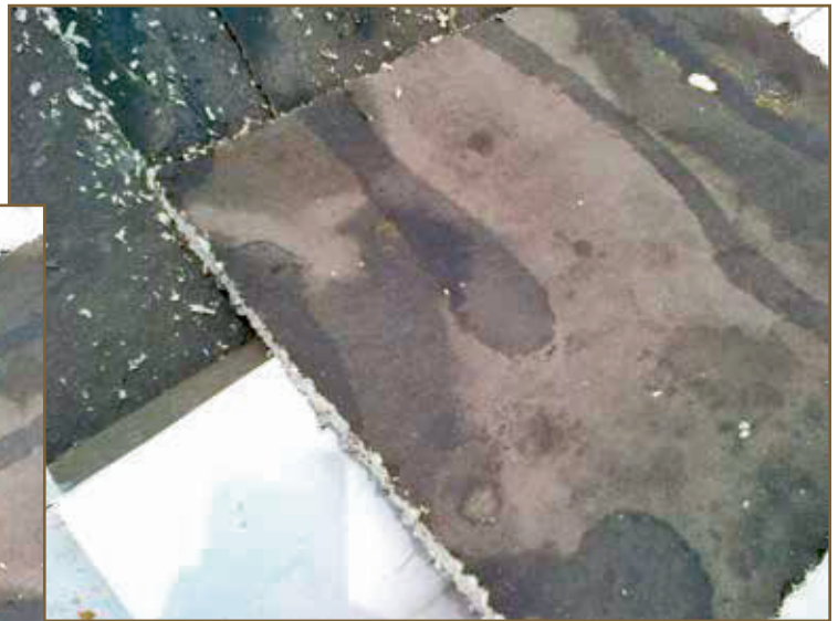
Photo 9 – Moisture between the layers of boards.
