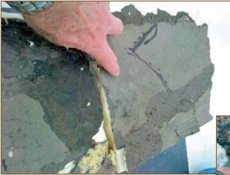
Photo 7 – Moisture underneath the bottom layer of iso.
