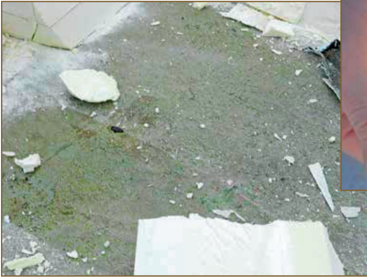
Photo 4 – Moisture on the deck; minimal primer.
