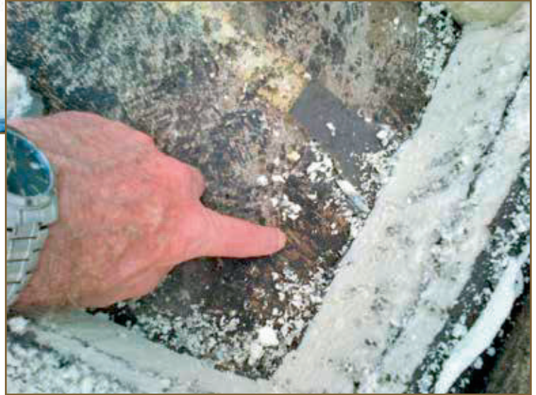
Photo 8 – Moisture on concrete deck.
