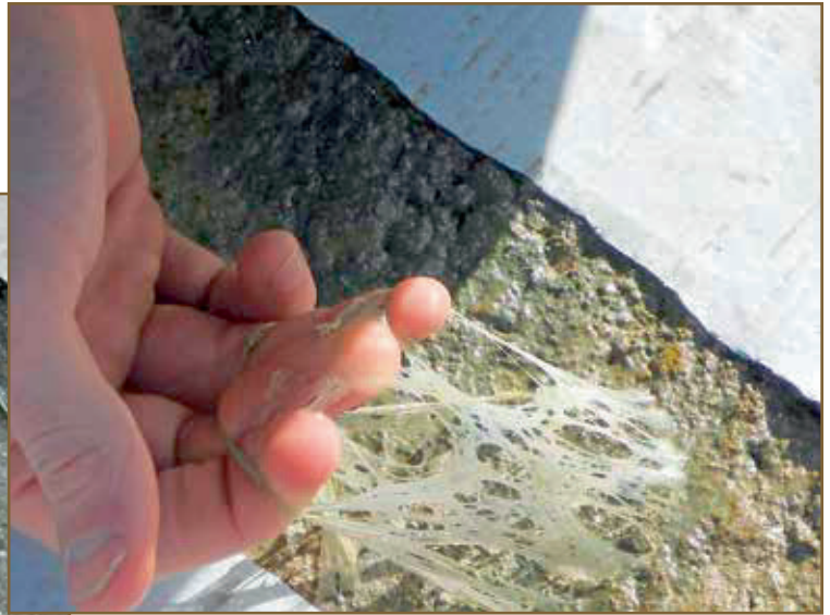
Photo 5 – Primer coming off the concrete deck.
