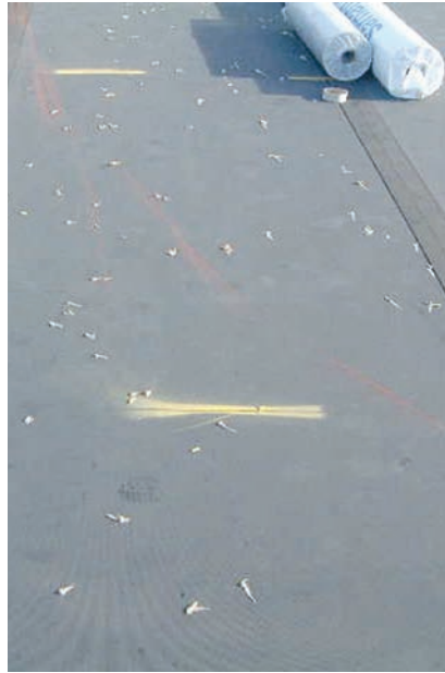
Advanced oxidation and loss of thickness of the exposed TPO membrane surface caused thousands of tiny pin holes to appear around the reinforcement scrim. To speed the installation process, grey caulking was used to cover many of the pin holes before the Sarnafil membrane was installed. The yellow lines were used to mark areas of the TPO that were leaking.
