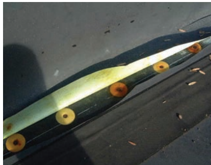
After only six years, the steel fasteners used to secure the former TPO membrane were rusted due to water infiltration through thousands of tiny pin holes that had been developed.
