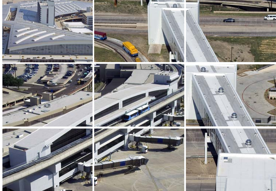
Sarnafil membrane was installed on Terminal D, the Grand Hyatt Hotel, the Skybridge and the Automated People Movers at Dallas/Fort Worth International Airport, Dallas, TX.
