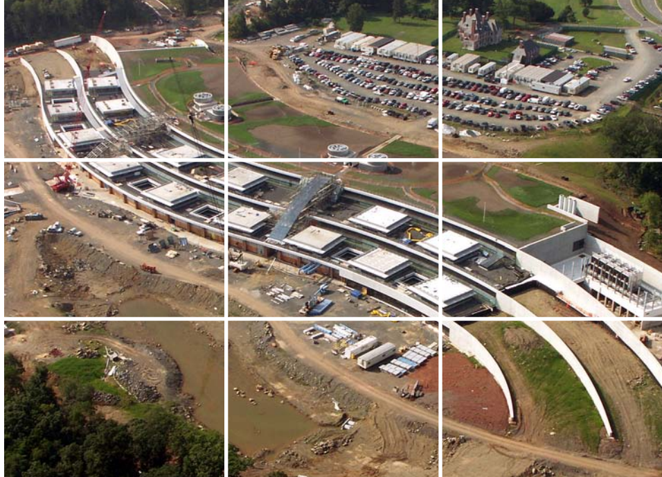
Seen under construction above is the Howard Hughes Medical Institute's Janelia Farm Research Campus. The Institute is home to a broad range of scientific programs aimed at advancing the study of biology and medicine.
