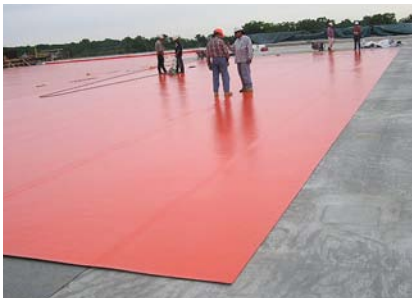
A section of waterproofing membrane is loose-laid over one of the Janelia Farm laboratories.
