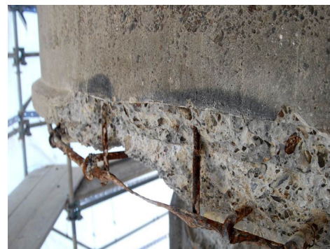
Concrete cornice with delaminated concrete
