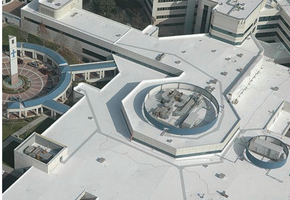
DRI installed the EnergySmart Roof on St. John's while the facility was open and operating. This prompted an accelerated schedule, and DRI employed a full-time Site Superintendent / Manager along with approximately 70 roofing and demolition workers.
