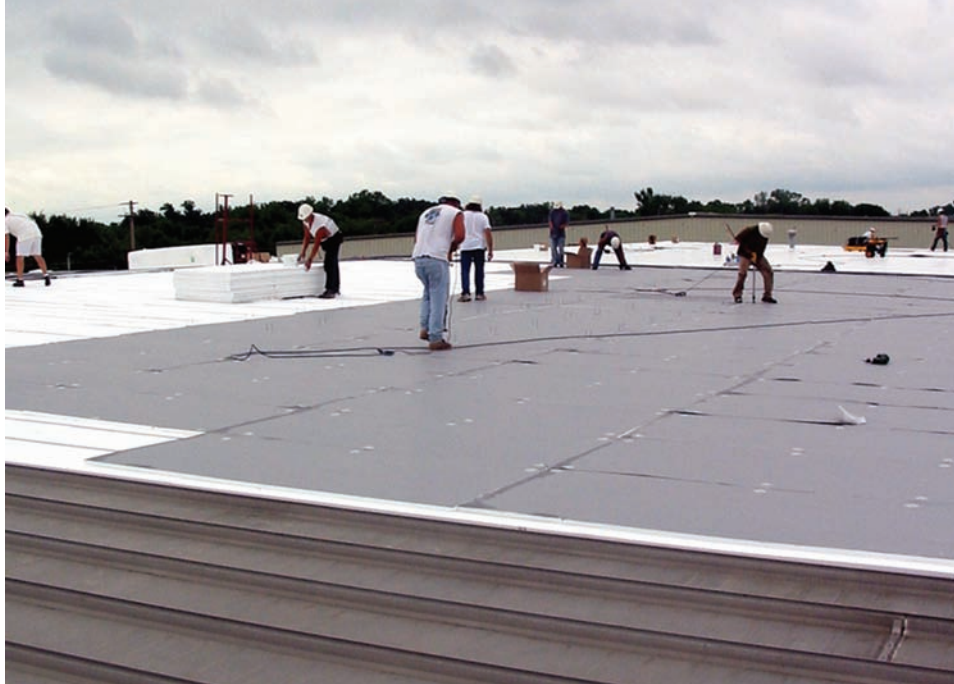
Premer Roofing employees fasten the cover board over the EPS flute filler.
