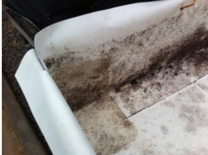
FIGURE 7. SARNAFIL G 410 MEMBRANE SURFACE AFTER THE MEDIA AND PLANTS WERE REMOVED. SOME MEDIA AND SOME FINE ROOTS STUCK TO THE SURFACE HOWEVER THEY WERE EASILY WASHED OR RUBBED OFF. SOME STAINING WAS OBSERVED.
