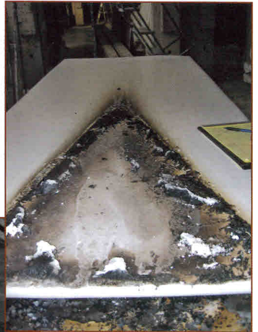
Photo 6 – PVC over listed gypsum board.
