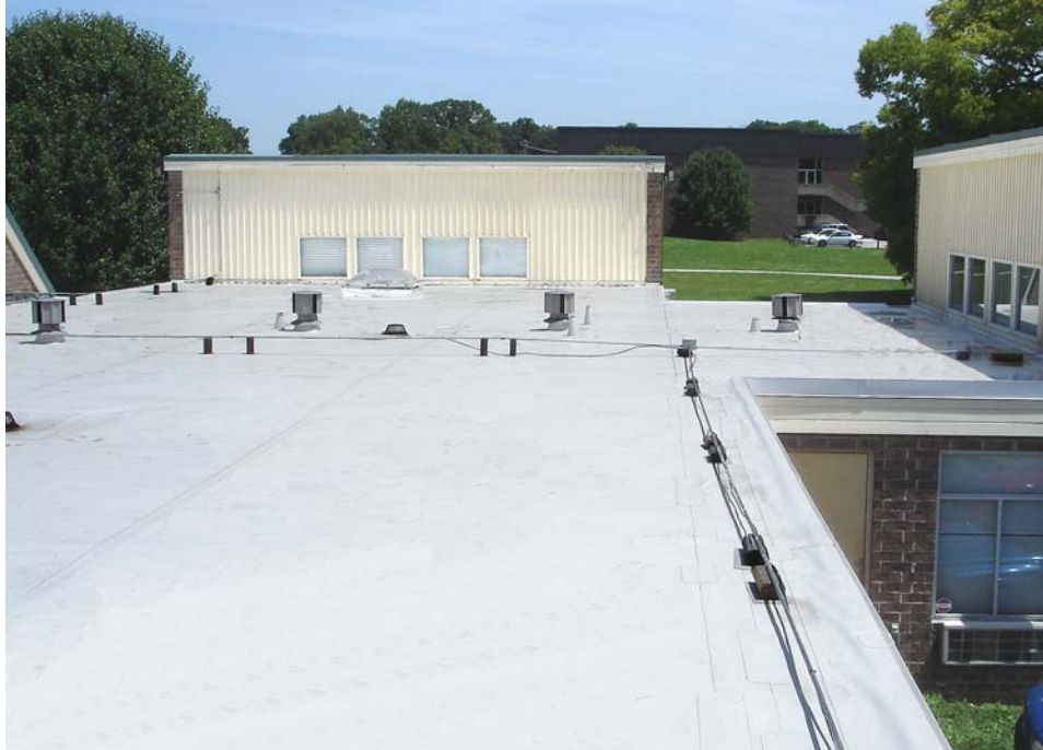
The numerous buildings at the Orange Grove Center utilize a wide variety of roof decks. Sika Sarnafil’s EnergySmart Roof (pictured above) was selected to cover low slope roof areas at the complex due, in large part, to the membrane’s versatility and energy efficiency.
