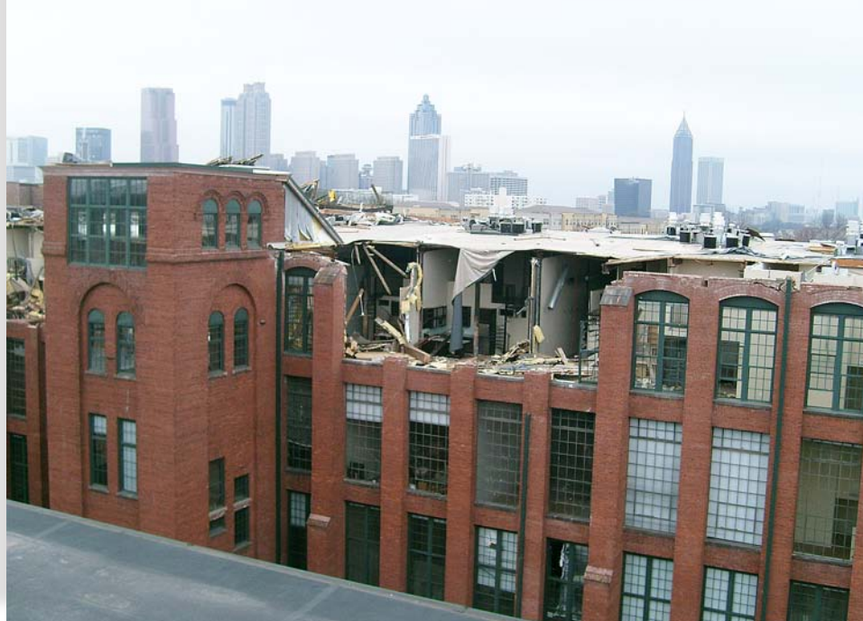
Stark evidence of the destruction tornados caused at the Fulton Cotton Mill Lofts in Atlanta in March, 2008. Roofing contractor T.L. Gowin installed new roofs on eight buildings within the complex totaling some 150,000 square feet.
