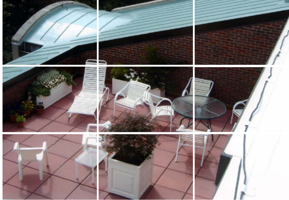
Luxury Condominiums patio deck, sloped and flat roof all utilize Sarnafil membranes.
