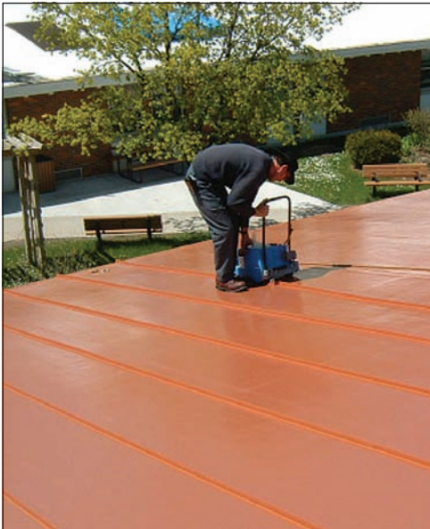
Worker fuses Décor Profiles to membrane using Sika Sarnafil's own Sarnamatic hot-air welder.
