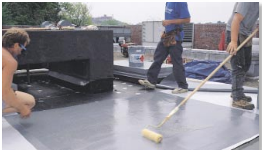
A PVC roof system being fully adhered. (Photo courtesy of Sarnafil Inc., Canton, MA.)
