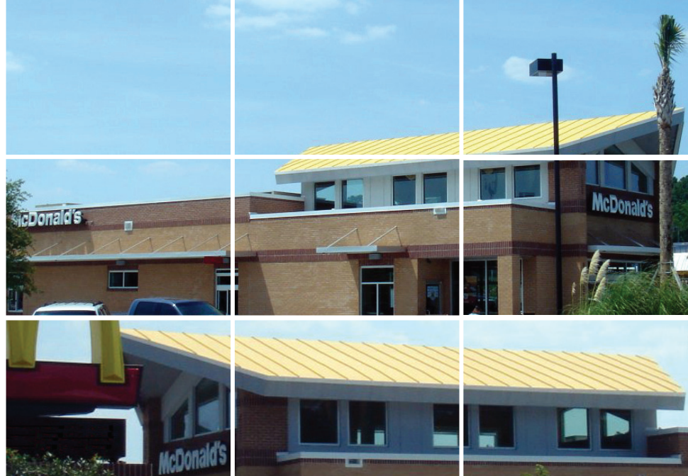
The Sarnafil Décor Roof System in custom yellow on top of McDonald's in Savannah, Georgia
