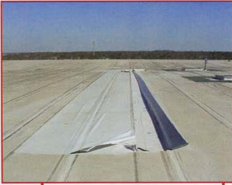
Photo 6: Membrane slit by a tumbling exhaust unit.
