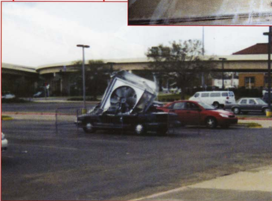
Photo 3: Exhaust unit blown off the roof.
