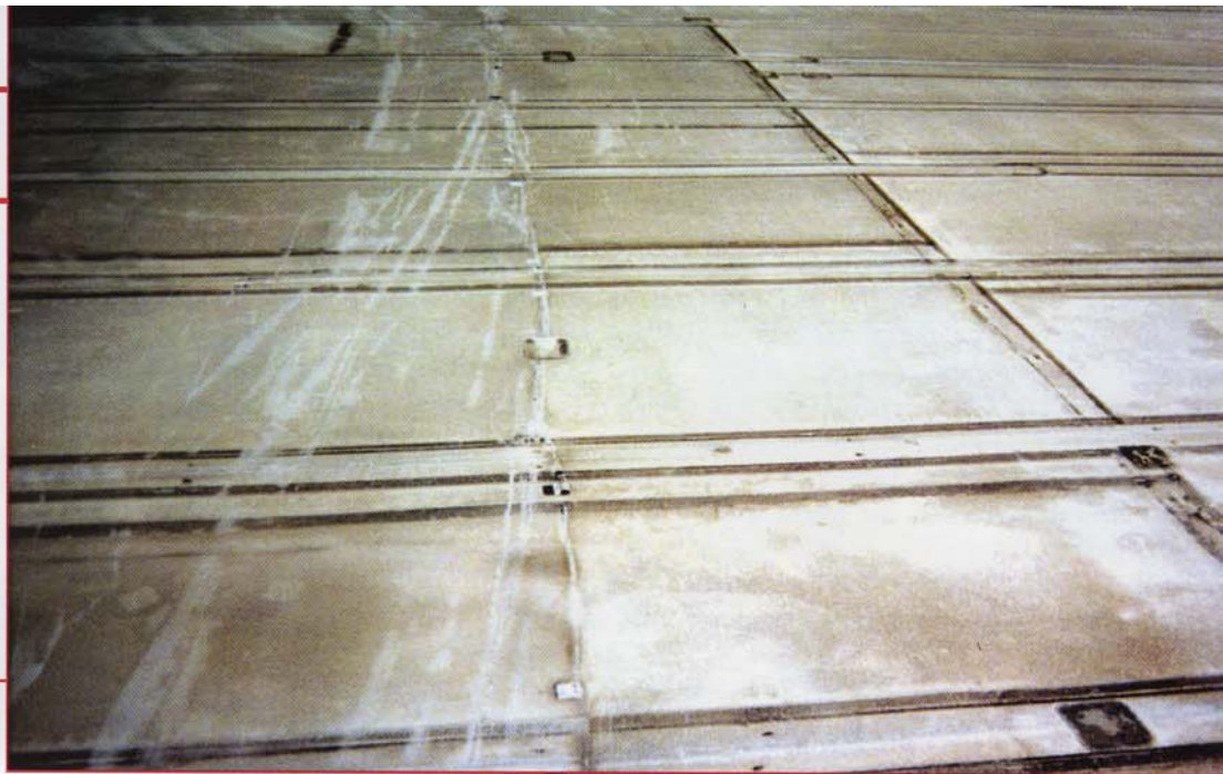
Photo 2: "Track" of one of the wind-blown HVAC units.
