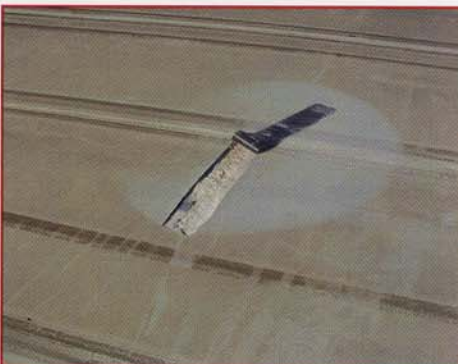
Photo 4: Membrane cut by an exhaust unit.
