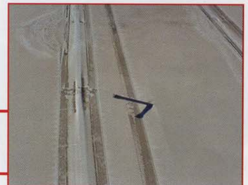
Photo 5: Membrane punctured by an exhaust unit.
