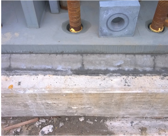
Figure 1: Figure 1: Shoulder cracking on SikaGrout® 928 installation
