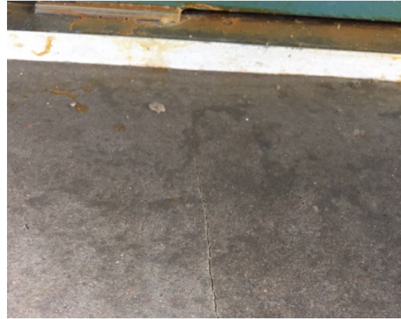
Figure 3: Shoulder cracking on SikaFlow® 648 installation
