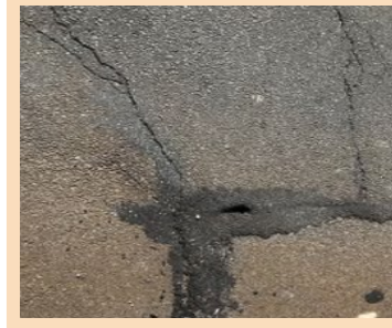
Stress causing damage
