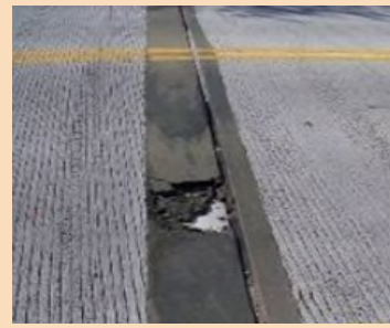
Poor bonding or delamination
