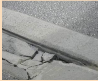
Surface depression or cracking
