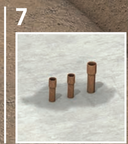
Leaking penetrations, i.e., pipe penetrations
