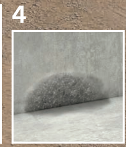
Leaking areas of voids, i.e., honeycombing
