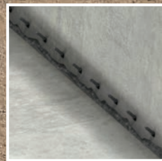
Leaking construction joints
