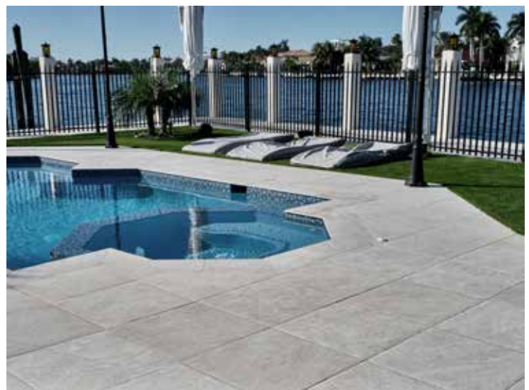
The Fort Lauderdale residence's extraordinary redesign demanded a full commercial construction system.
