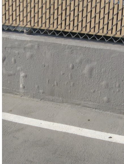
B. Excessive vapor drive
