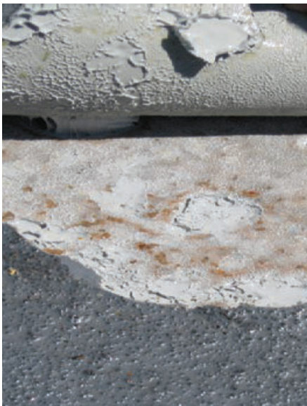
D. Improper mixing
