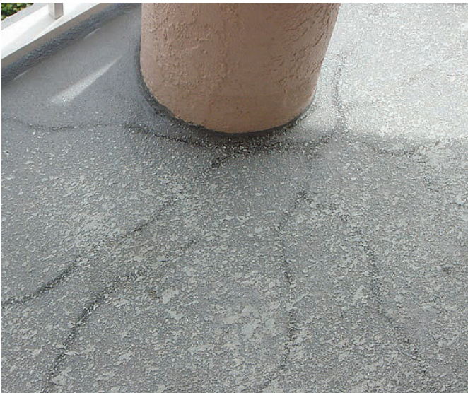
B. Improper sealant chemistry
