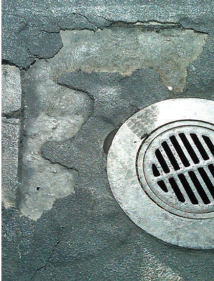
A. Improper concrete surface preparation
