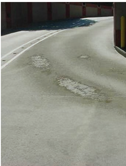
D. Incorrect System Selection
