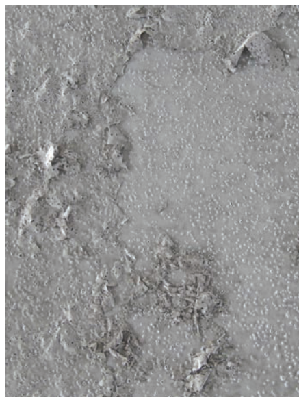
E. Improper surface preparation of existing coating
