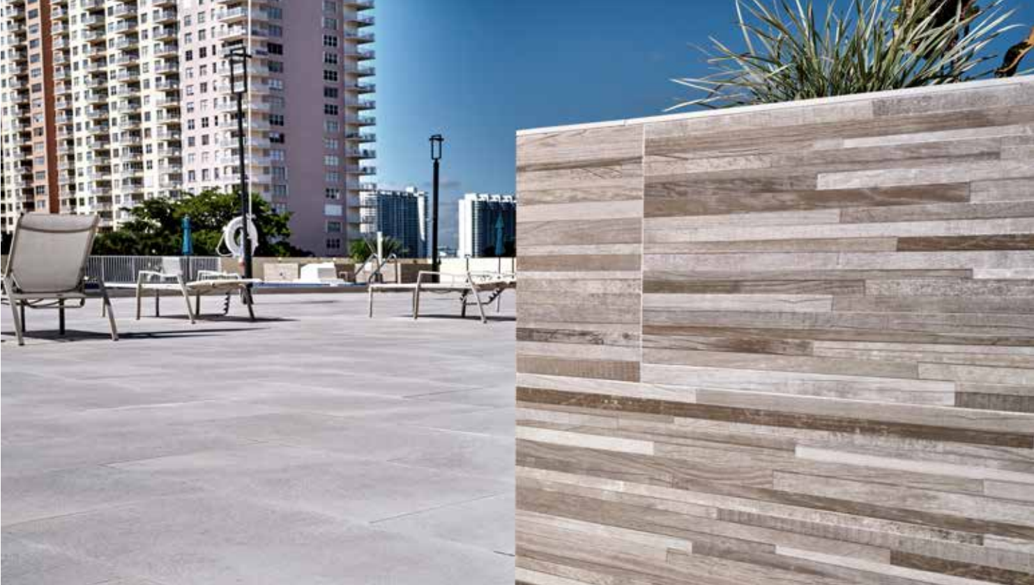
The amenities area received a new porcelain deck and wood-look mosaic planters.
