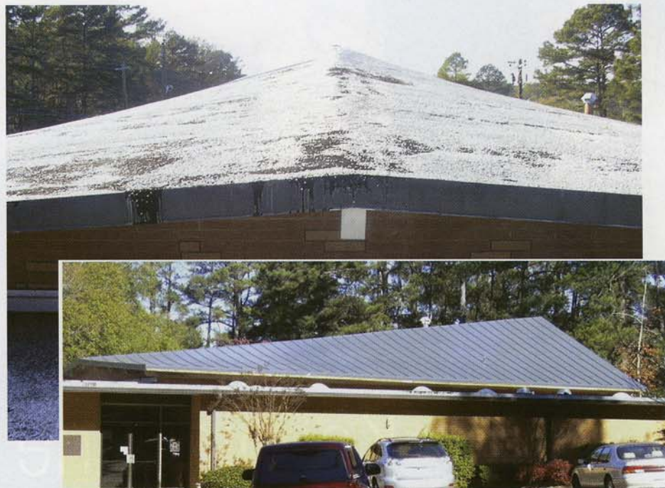
Top: The temple’s built-up roof system before the tear-off Bottom: The new PVC membrane roof system Photos courtesy of Thomson Roofing and Metal Co., Thomson, Ga.
