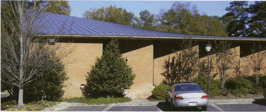
The seams on the temple project needed to lay parallel to the slope to accommodate the décor ribs.
