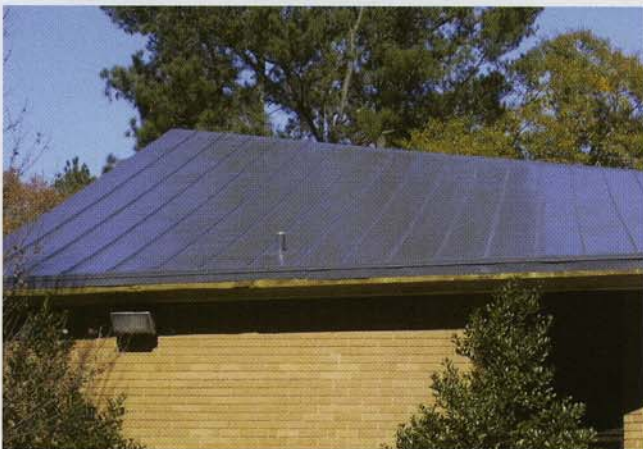
The PVC membrane roof system was chosen for its metal appearance and ability to accommodate the roof line.
