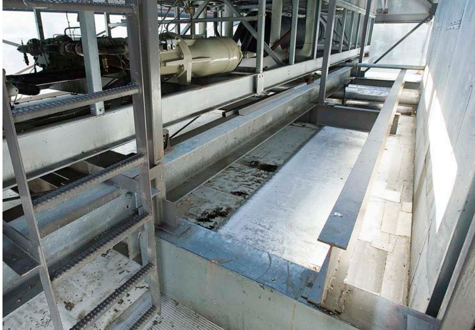
A look "inside" the massive HVAC unit suspended just above the roof at the Munson Medical Center. Bloxsum Roofing had to contend with the unit's stairways, suspended walkways and wall built for soundproofing.
