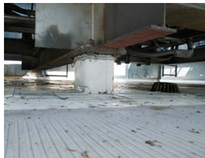
Close quarters forced Bloxsum Roofing workers to complete much of the work while lying on their stomachs.
