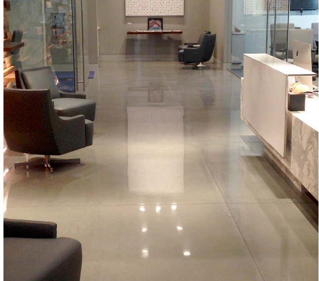
ALEXANDRIA CENTER A smooth, consistent gray finish for their office floors was requested by this client. Their vision was achieved using Sika® Formula One™ Lithium Densifier MP, Sika® Formula One™ Finish Coat and Sika® Formula One™ Liquid Dye Concentrate in "Concrete Gray".
