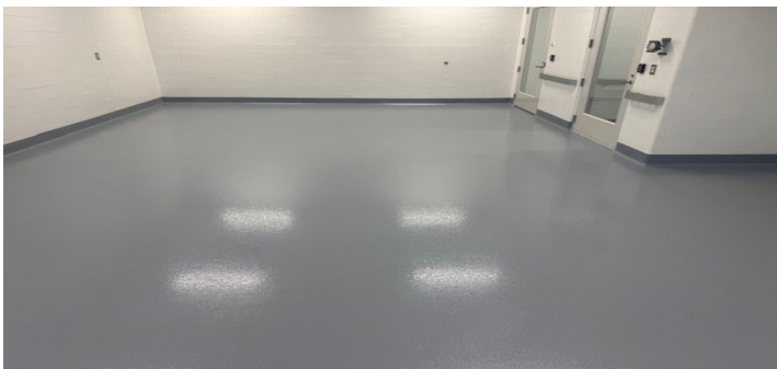
BSL-3 clean room with seamless floor-to-wall transitions.
