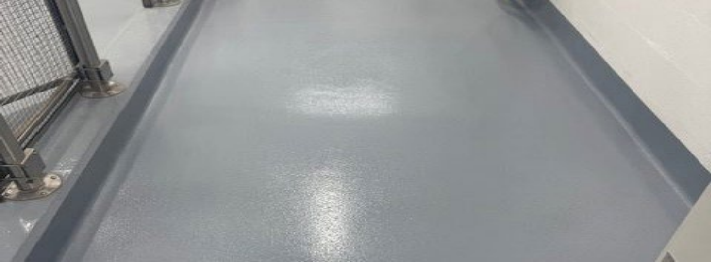
BSL-3 holding area featuring Sika Ucrete seamless flooring with containment equipment.
