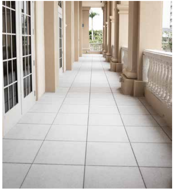
SikaTile®-815 Secure Grout retains its flawless appearance after Hurricane Ian flooded the Ritz-Carlton.
